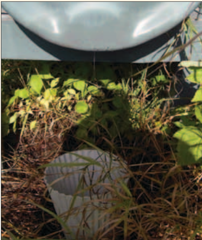
Leaking oil tank. Note the steady stream of oil from a pin-hole leak.
