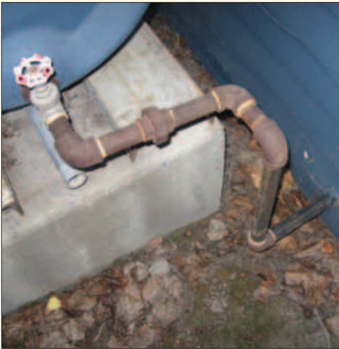
This type of fuel line is called a swing joint, which accounts for tank movement.
