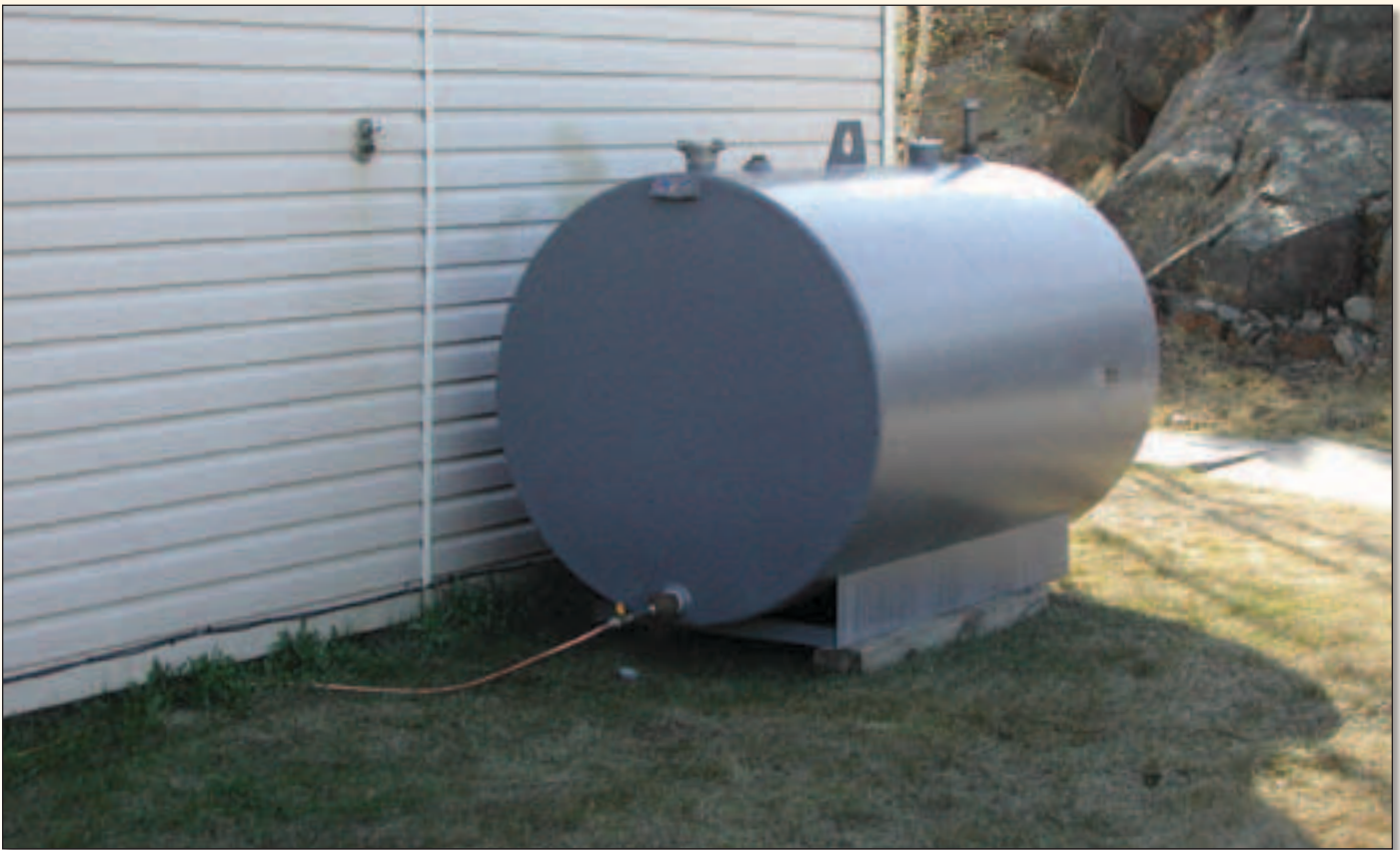
Double-wall steel heating oil tank.
