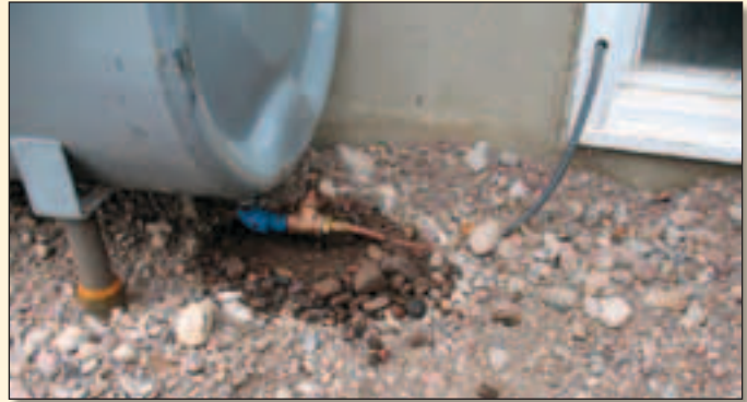
Small spill from a leaking valve.
