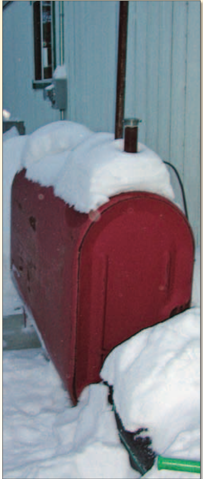
Typical oil tank location.
