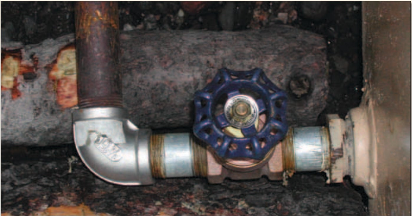
Newly installed oil tank valve. Note the oil stained ground still requiring clean-up.
