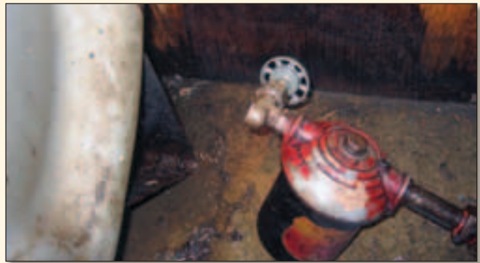
Broken valve on oil tank in basement.
